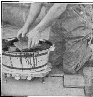
(2) Hold block horizontal and dip bottom in EVERBOND to a depth of 1/8 in. This will give the under side, including the hollow-backs, an even coat of EVERBOND without touching the tongue or grooves.
